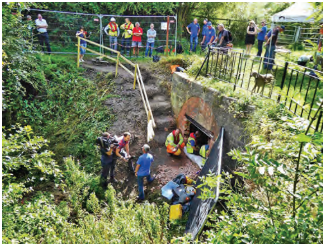
BBC Look North interview taking place. The temporary steps built by the contractors are seen. Photo John Lower
